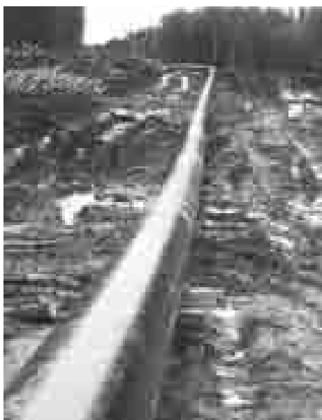
Installation of Shell's Sakhalin II pipeline slashing through a forest. (Sakhalin Environment Watch)
